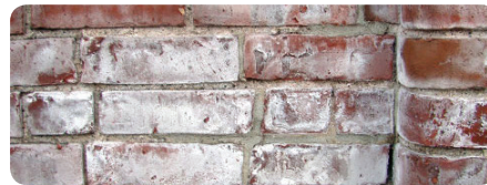
Masonry surface: Brick walls/concrete slabs subjected to damage from moisture/efflorescence
